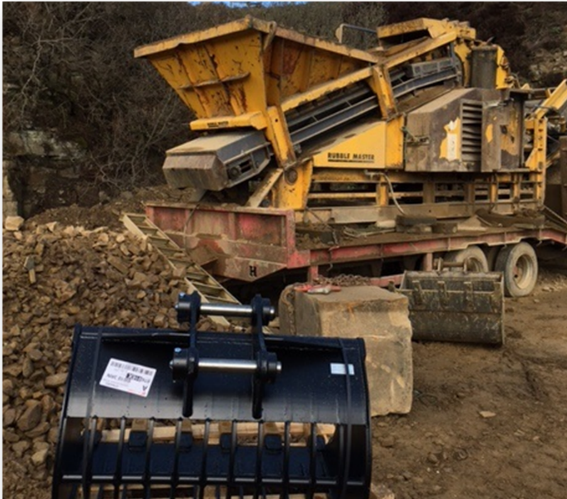
Catlow East crushing plant
